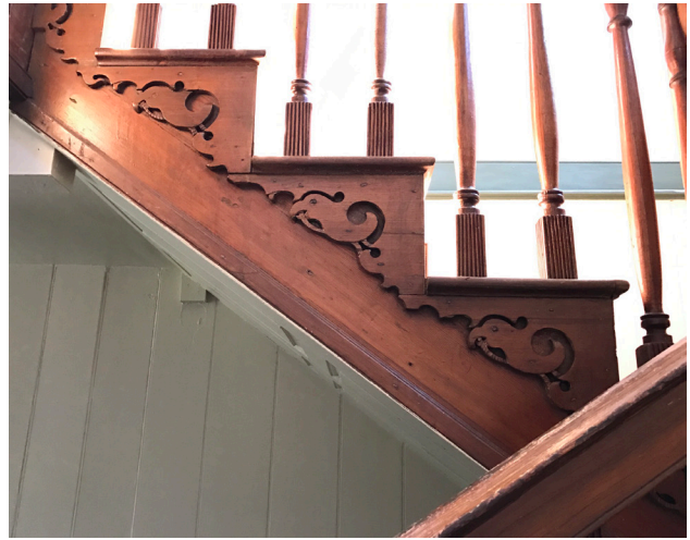
Figure 10. The main stairway, connecting the lower and upper halls, is also beautifully carved, decorated on the end of each step with an Eagle holding an olive branch.
