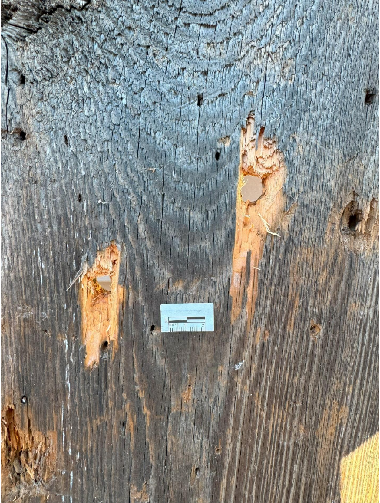
Figure 17. Exit holes on the interior wall paneling of Wall 1.
